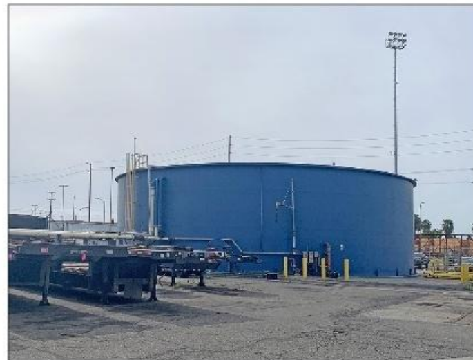
Aboveground Storage Tank
