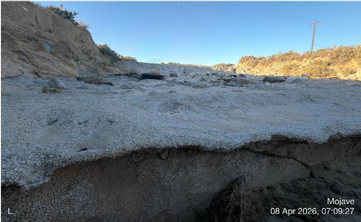
Photo 2. View of eroded apron from Turner Road to the scour point
