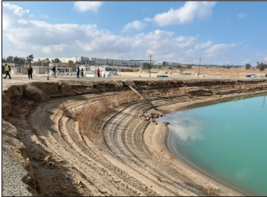
Figure 2: RW Storage Pond Severely eroded slope
