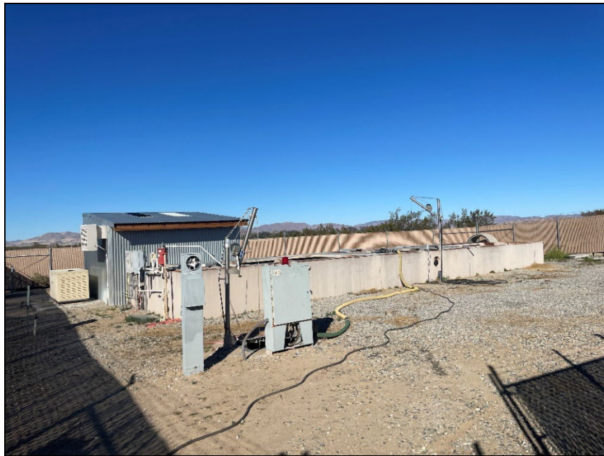
Figure 5. Fenced Enclosure with Structures (view northeast; December 10, 2025).
