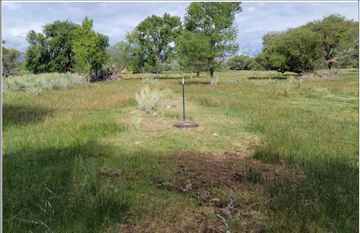
Photograph 8: Photograph depicts ESCSD Collection System Segment between South Barlow Lane and Sunland Drive where ESCSD Collection System parallels Sunset Drive, facing west (Taken on 05/28/2026).
