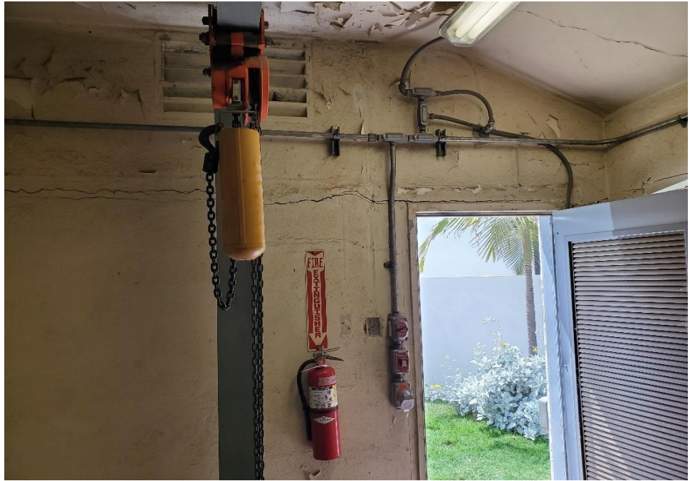
Photograph 13: Horizontal crack on the upper floor of the lift station, above the doorway on the southeast wall of the building, looking southeast.
