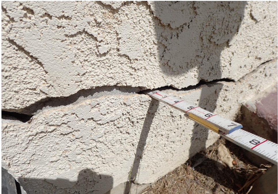
Photograph 10: Close up of 2-inch-deep crack on the south corner of the building in photograph 7.
