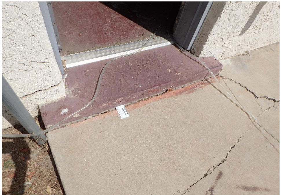
Photograph 4: Separation between the building entrance and the sidewalk.
