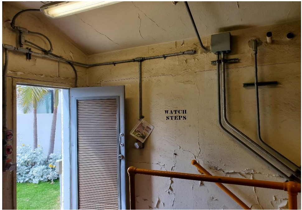
Photograph 15: Horizontal crack on the upper floor of the lift station, on the southwest wall of the building, looking south.
