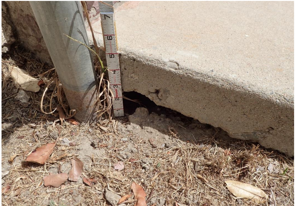
Photograph 8: Close up of 2½ inches of separation between sidewalk and ground surface in photograph 7.
