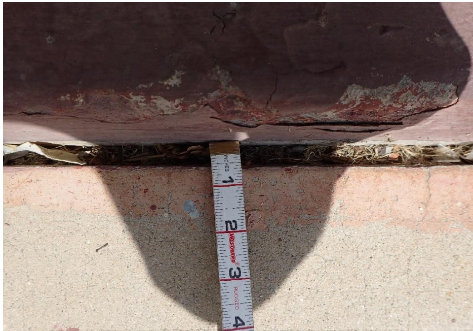
Photograph 5: Close up of 1/2-inch horizontal separation in photograph 4.
