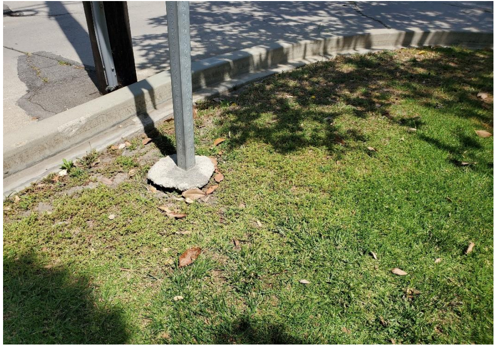
Photograph 11: Settlement of the ground surface around a street sign on the north corner of the property, looking north.
