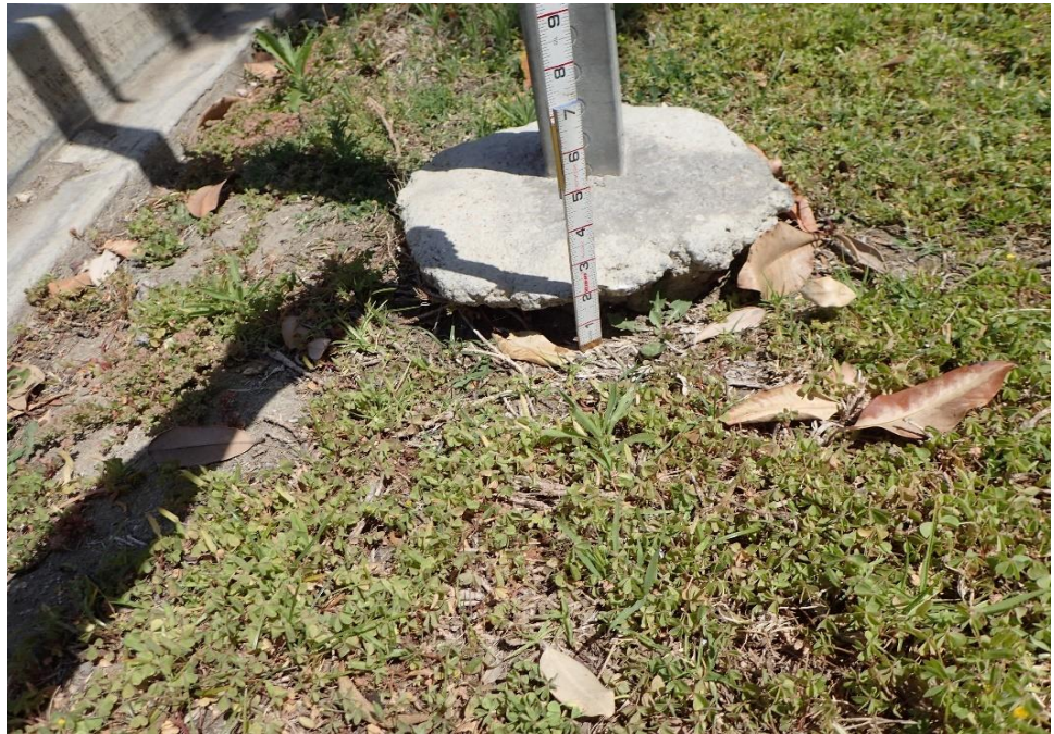
Photograph 12: Close up of 2 inches of settlement of the ground surface in photograph 11.
