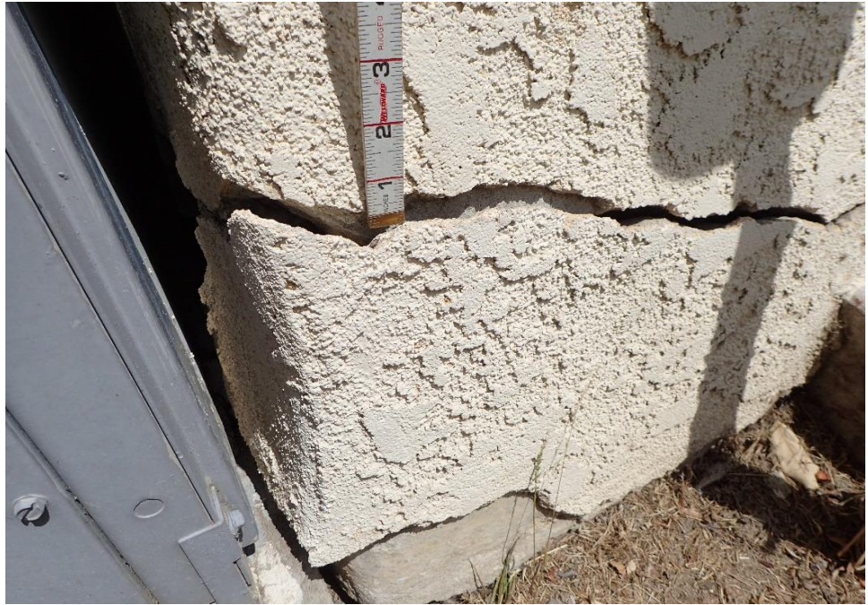
Photograph 9: Close up of ½-inch-wide crack on the south corner of the building in photograph 7.
