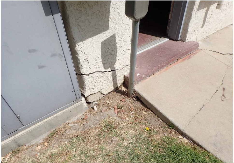
Photograph 7: A crack on the south corner of the building was noted, as well as a vertical separation between the sidewalk and the ground surface.
