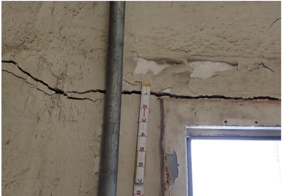
Photograph 14: Close up of 1/4-inch-wide crack in photograph 13, above the doorway on the southeast wall of the building.
