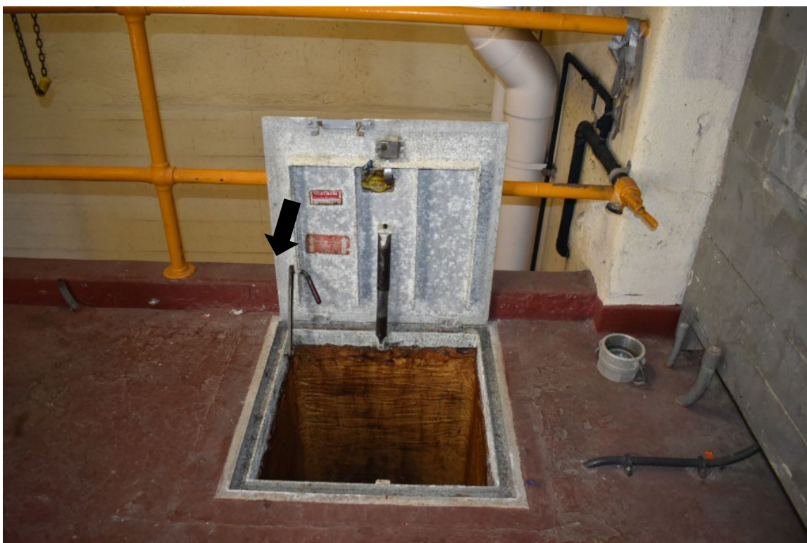
Figure 16. Wet Well Check Plate/ Access (Superstructure Interior)
