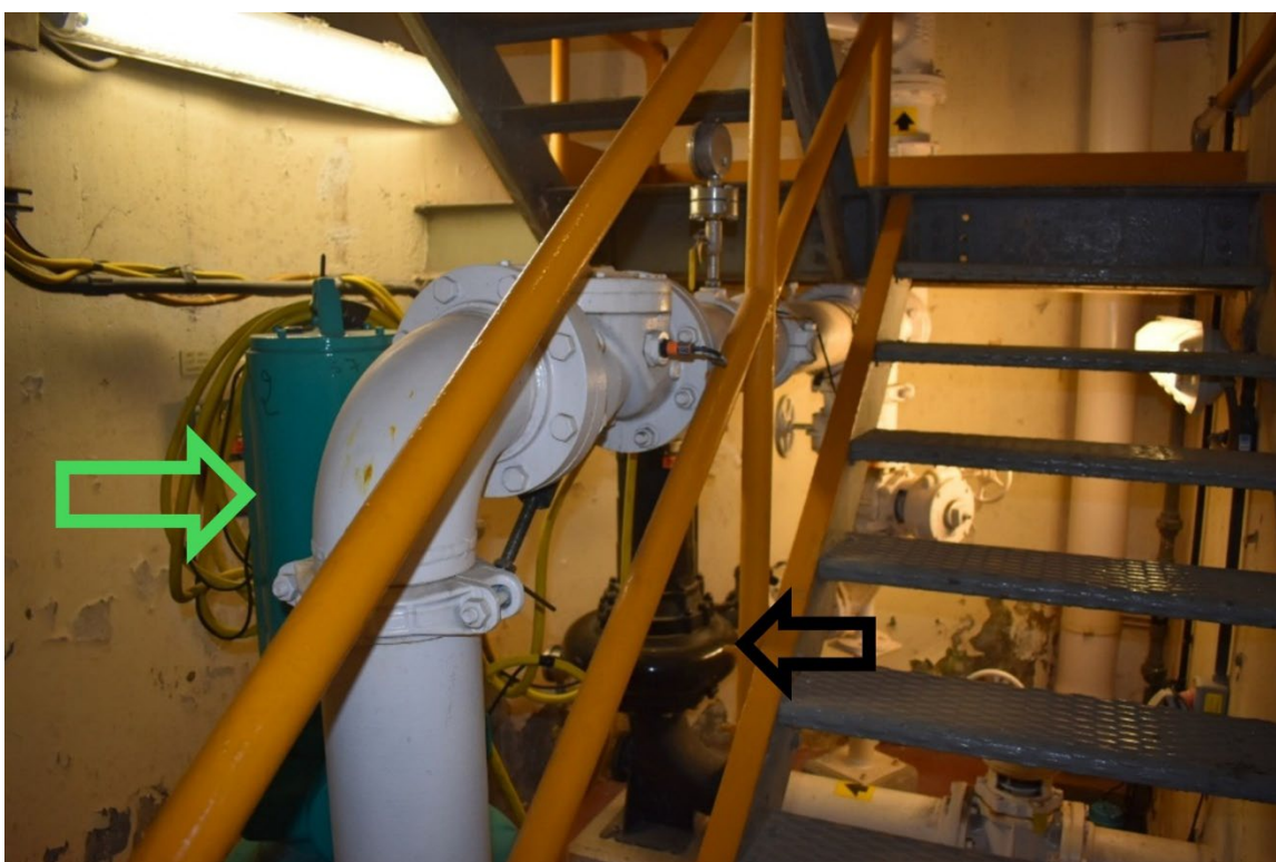
Figure 17. Basement, Pump No. 1 Motor (Black) and Pump No. 2 Motor (Green)
