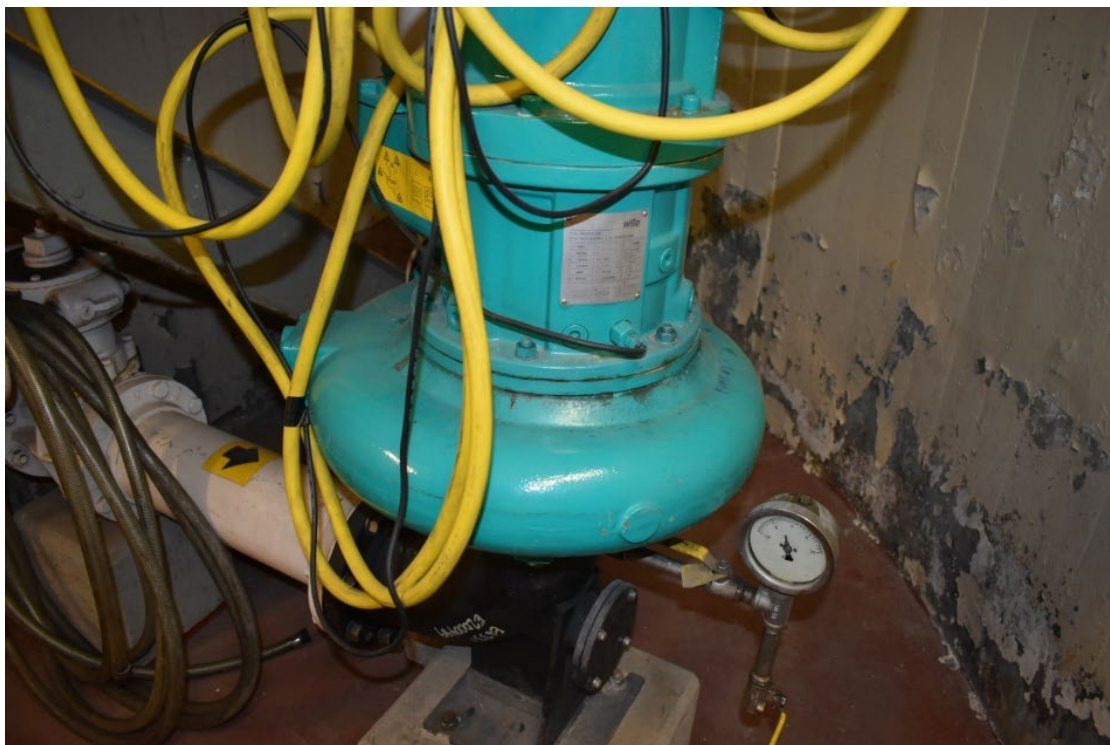
Figure 18. Basement, Detail of Pump No. 2 Motor
