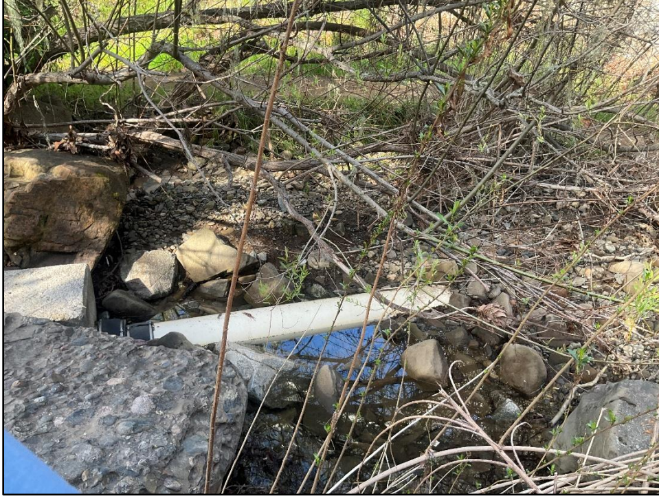
Photo 3. View east of concrete hold-down and exposed pipe in Atascadero Creek (03-02-2026).
