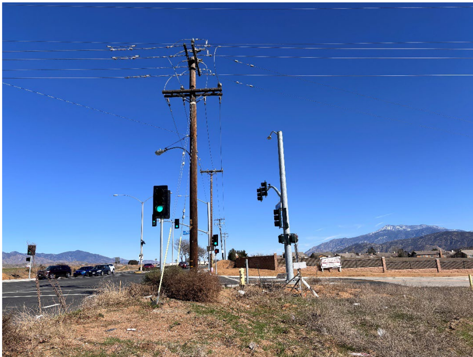
Photograph 4: P-33-023484/CA-RIV-23484, SCE Memphis 12kV Distribution Line. View to the east.
