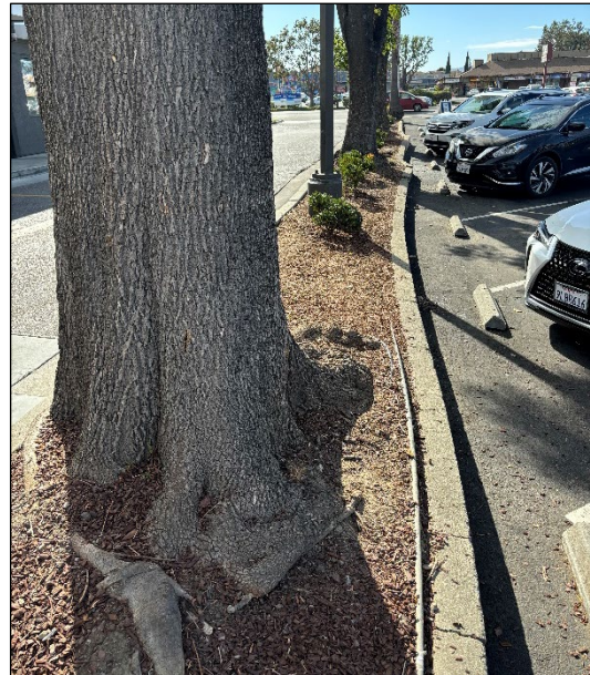
Photo 3: Significant curb displacement adjacent to trees #157, 158, and 159.
