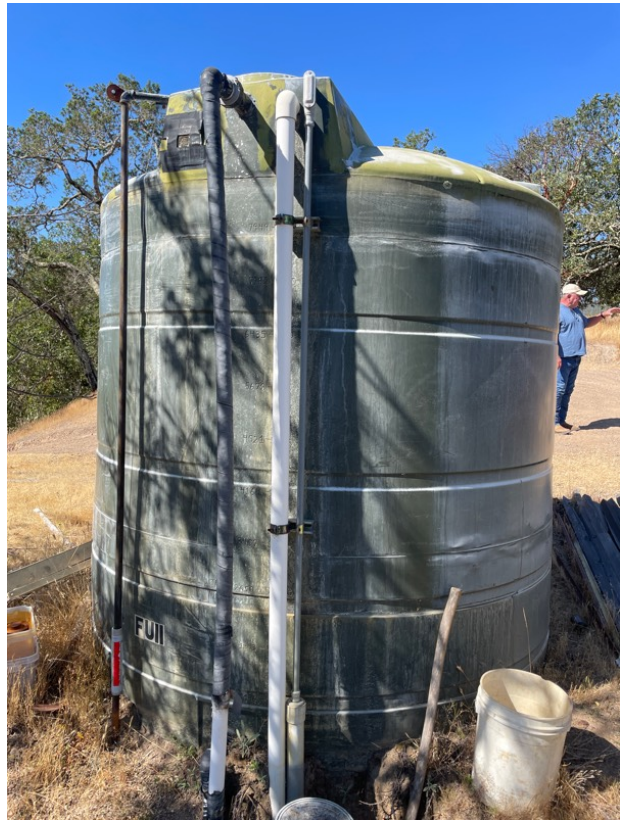
Polyethylene Storage Tank
