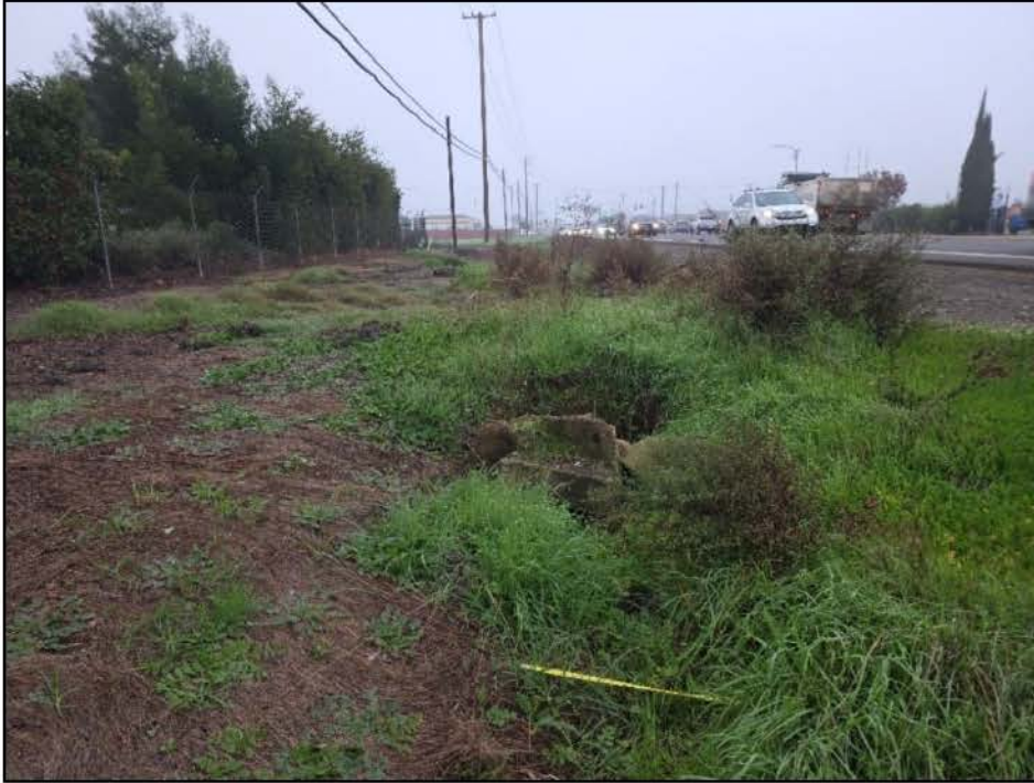
Photograph 15. Detail of damaged culvert, originally recorded at P-34-005400 in 2020, December 5, 2025.
