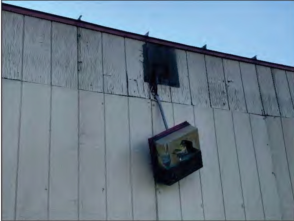
Photo 7. Hole on Exterior of Portable Building—Potential Entrance into the Interior. Potential Suitable Bat Habitat.
