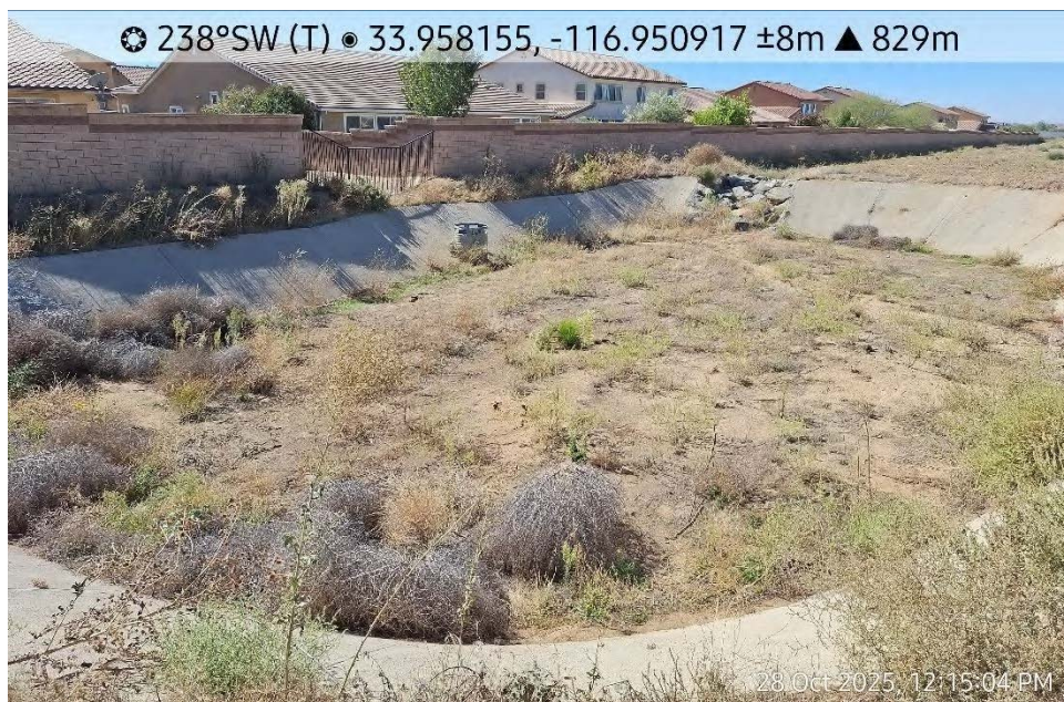
Photograph 6. View of modern water detention basin in southwestern corner of project site.
