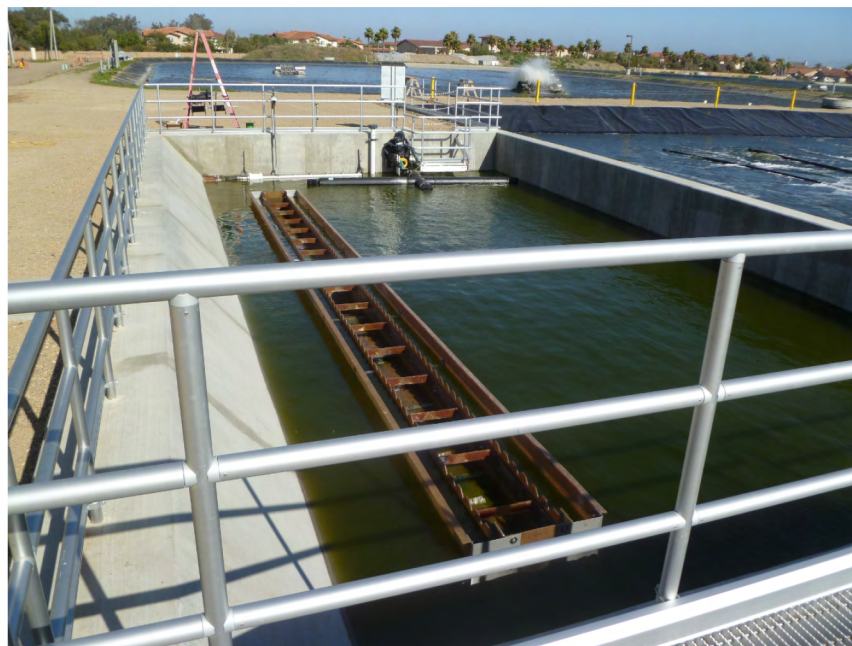
Figure 4-7 Photo of Integral Clarifier Prior to Startup (Courtesy of Parkson Corporation)
