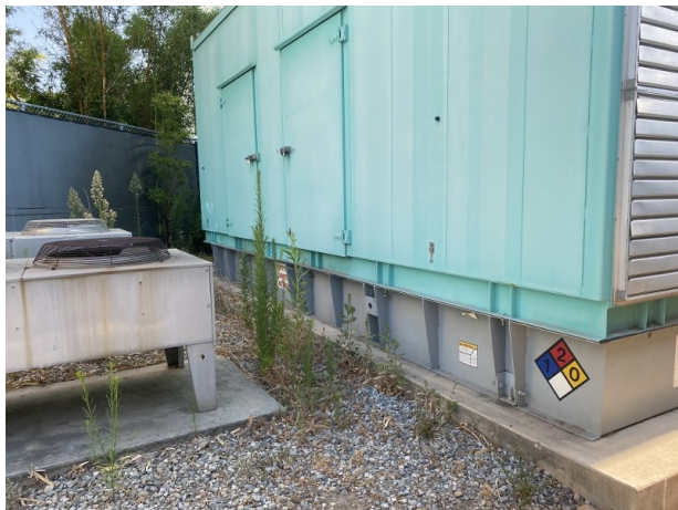
5.View of the subject property: backup generator
