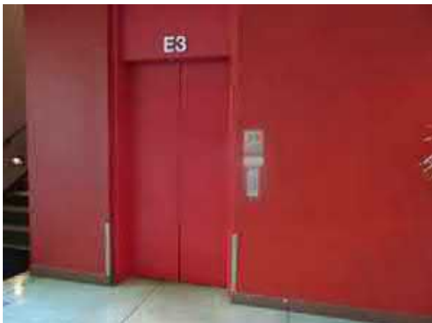
29. View of typical elevator on the subject property.
