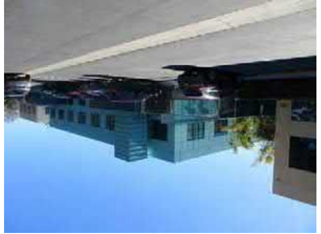
3. View of the systems cooling tower on the eastern portion of the subject property facing northwest.
