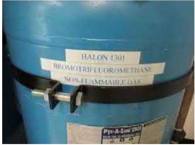
44. View of Halon 1301 fire suppressant located on the subject property.
