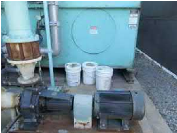
55. View of three five-gallon systems cooling tower routine maintenance treatment.
