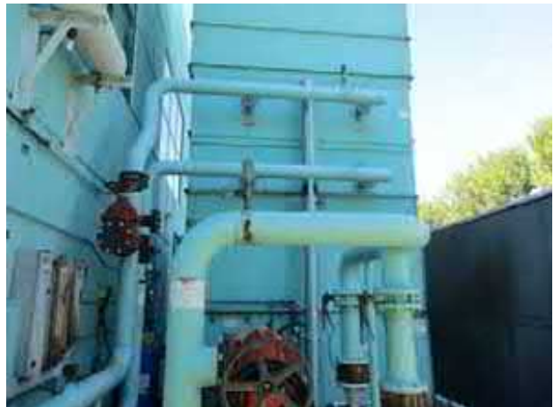
54. View of systems cooling tower located on the eastern portion of the subject property.
