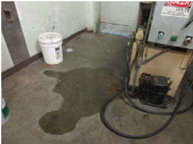
47. View of leak near trash compactor equipment.
