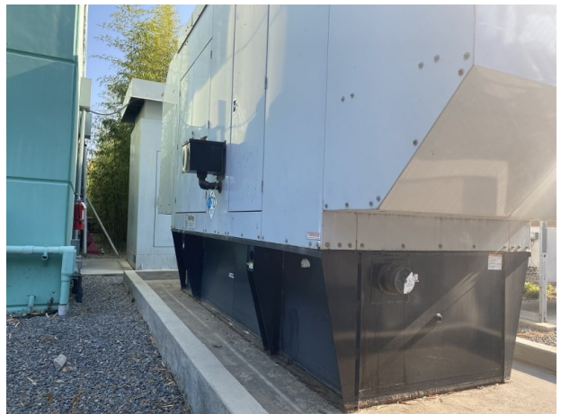
6.View of the subject property: backup generator
