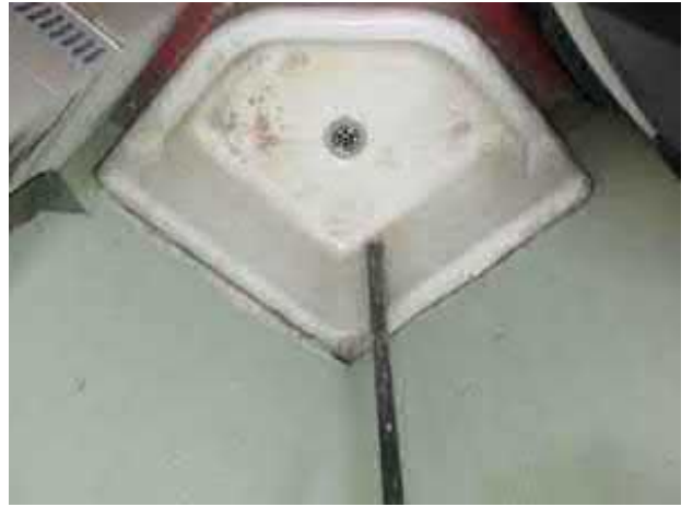
39. View of mop sink in the janitorial closet.
