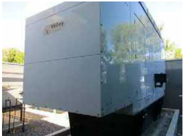
52. View of emergency generator located on the eastern portion of the subject property.
