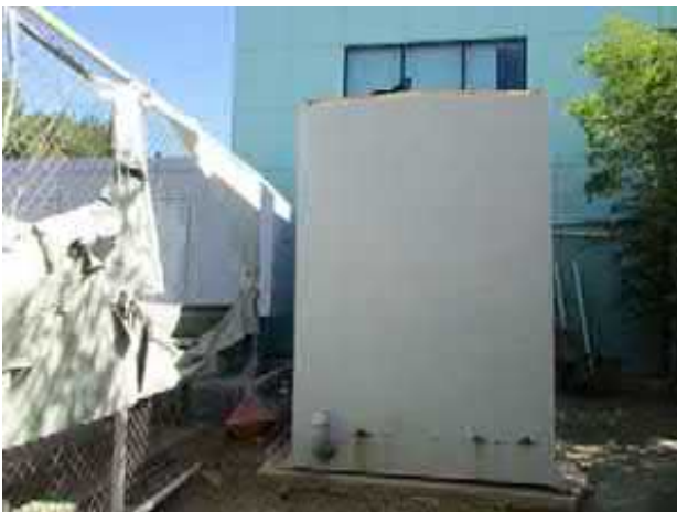
51. View of emergency generator located on the eastern portion of the subject property.
