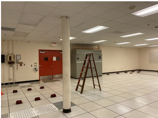
11.View of the subject property: server room
