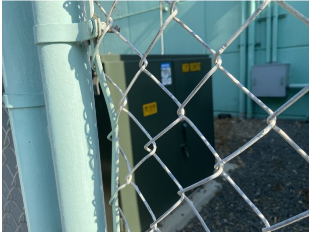
7.View of the subject property: transformer
