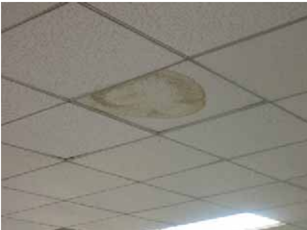
35. View of stained drop down ceiling.
