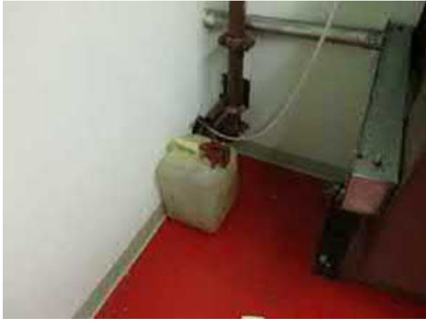
43. View of container located in address 2401B in elevator equipment room of the subject property.
