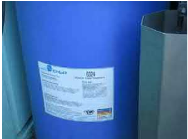
56. View of systems cooling tower treatment container located near the eastern portion of the subject property.
