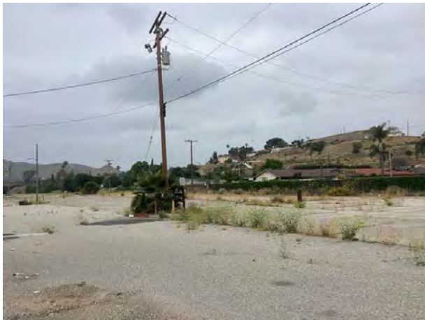
3 : View of the pole-mounted transformer
