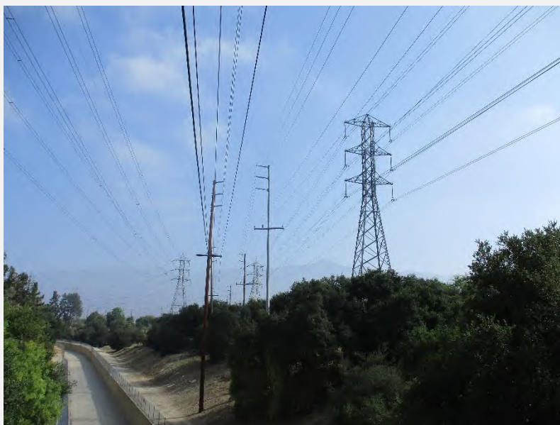
Photograph 17. The SCE Mesa-Anita-Eaton Transmission Line along the Eaton Wash Channel, looking northeast.
