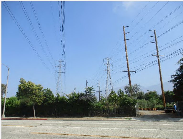
Photograph 1. The SCE Mesa-Anita-Eaton Transmission Line, looking south.
