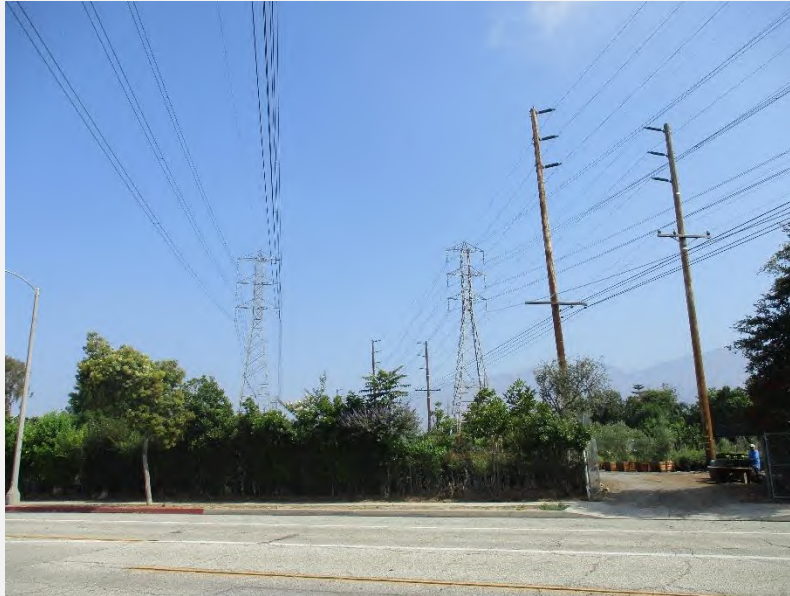
Photograph 16. The SCE Mesa-Anita-Eaton Transmission Line, looking south.
