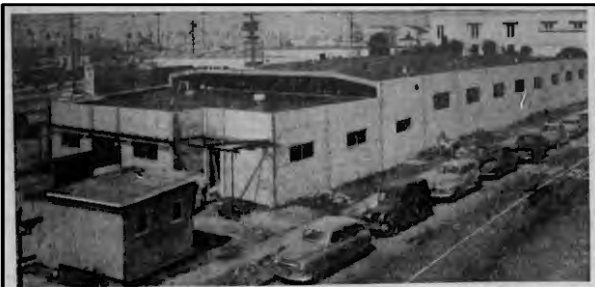
BEING BUILT —Shown above is new industrial plant now under construction at 4800 San Vicente Blvd. for Hollywood Clothes. Building contains 30,000 square feet of space and will cost, including land, approximately $300,000. Among the features is a complete boiler system for operation of steam pressing section. Project was designed by Donald R. Warren Co., engineers. Contractor is Chatiner & Gumbiner.
