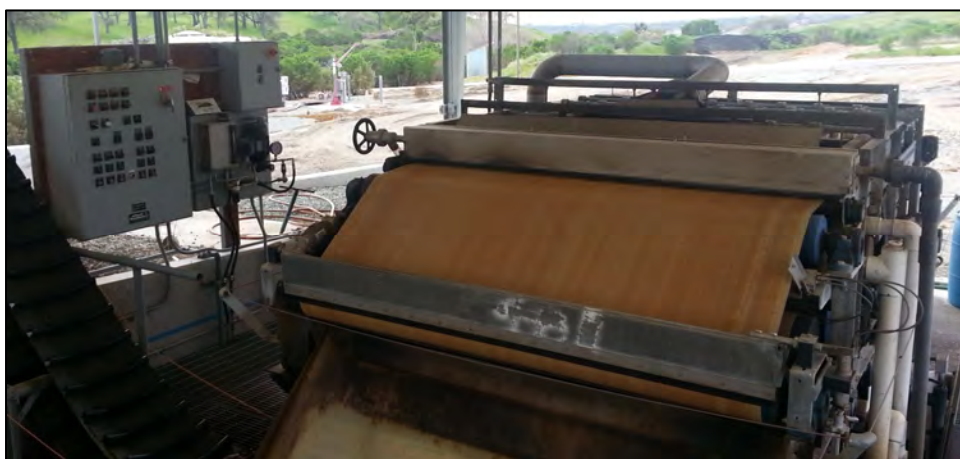
Photo: Biosolids Dewatering Filter Press
