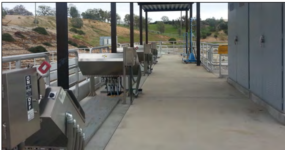
Photo: UV Disinfection System Channel
