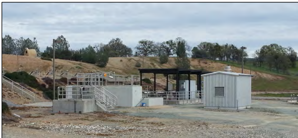
Photo: Tertiary Filters, Blower Bldg. and UV Disinfection System
