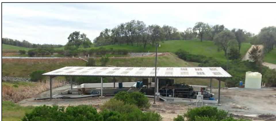
Photo: Biosolids Dewatering Facilities
