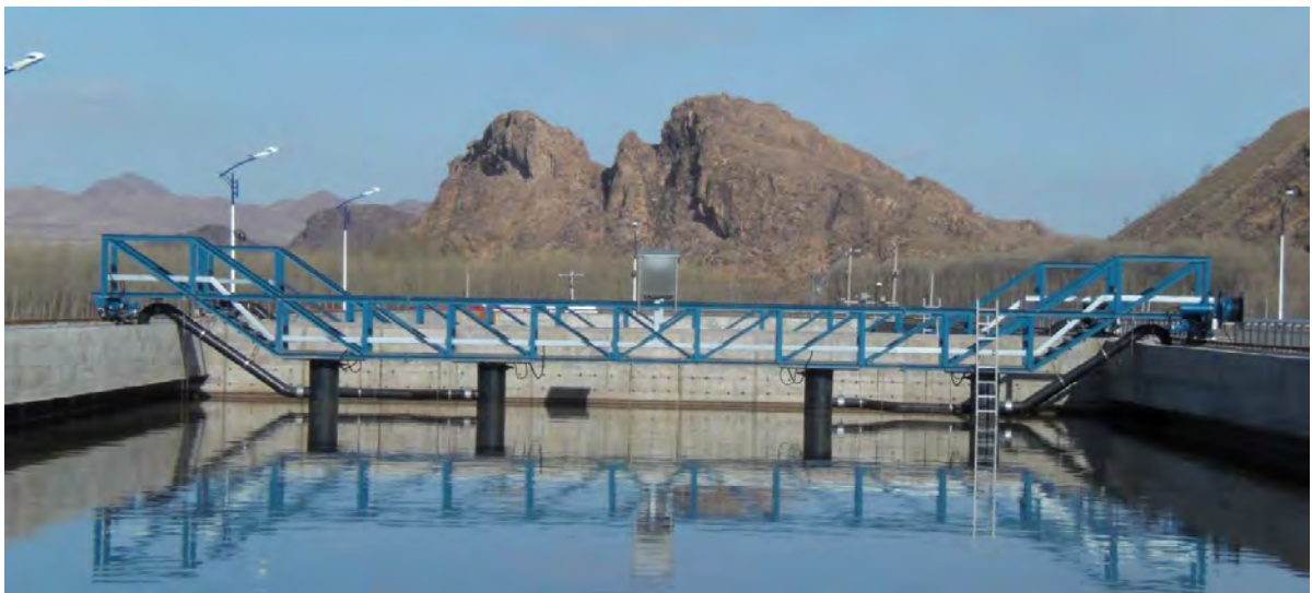
BIOWORKS® clarifier in operation
