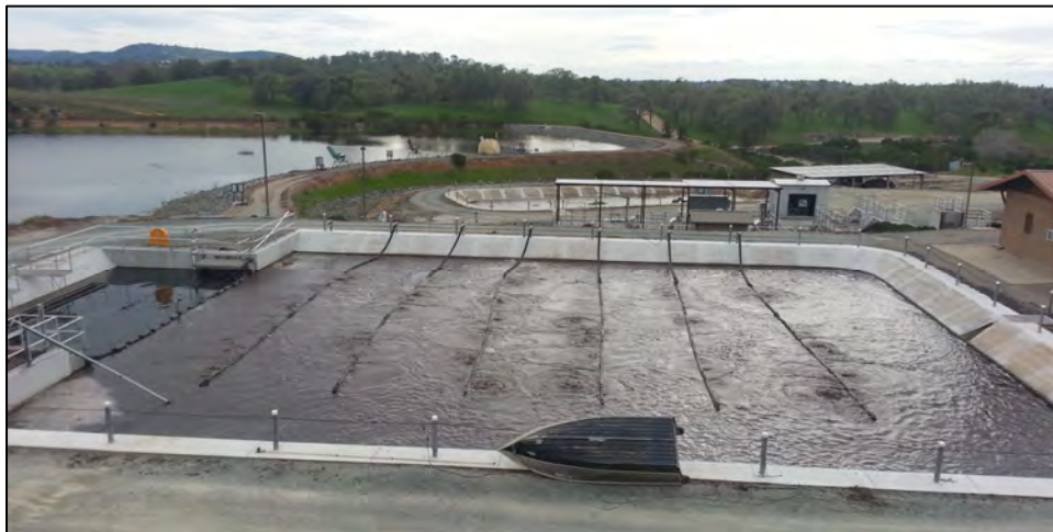
Photo: Existing Biolac® Basin and Clarifier
