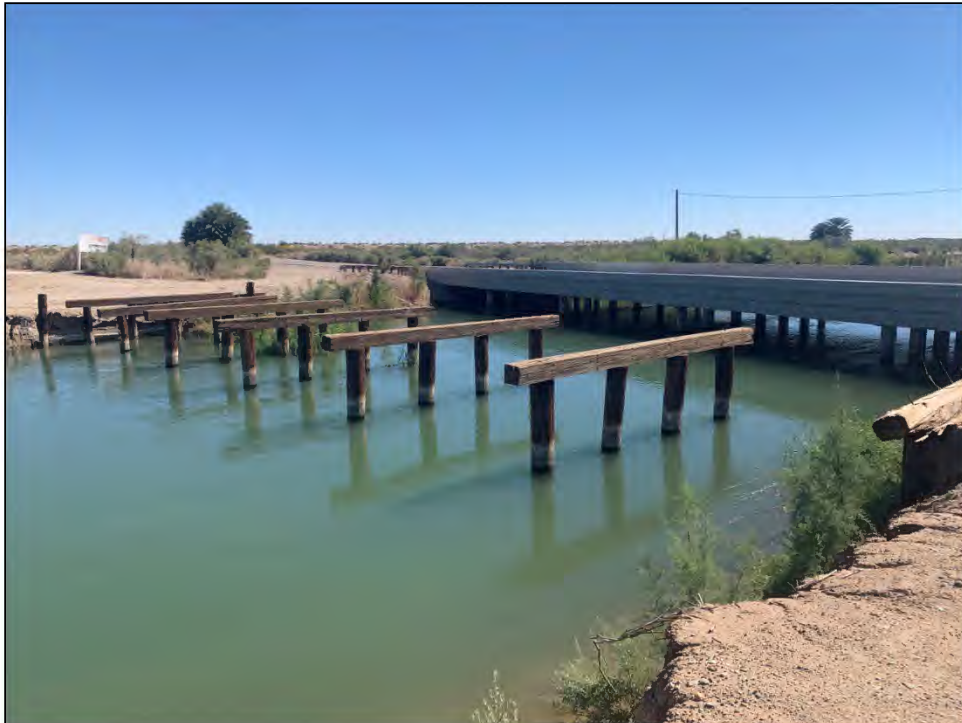
Photo 10: North side of SR-78 bridge crossing over the East Highline Canal; facing south.
