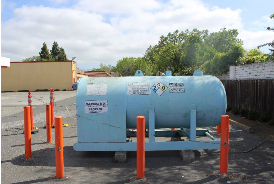
Photograph 8: 1152 Tully Road propane tank, camera facing northeast, April 23, 2025.
