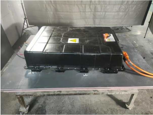
Figure 9 – Module on the test platform – Side view 1
