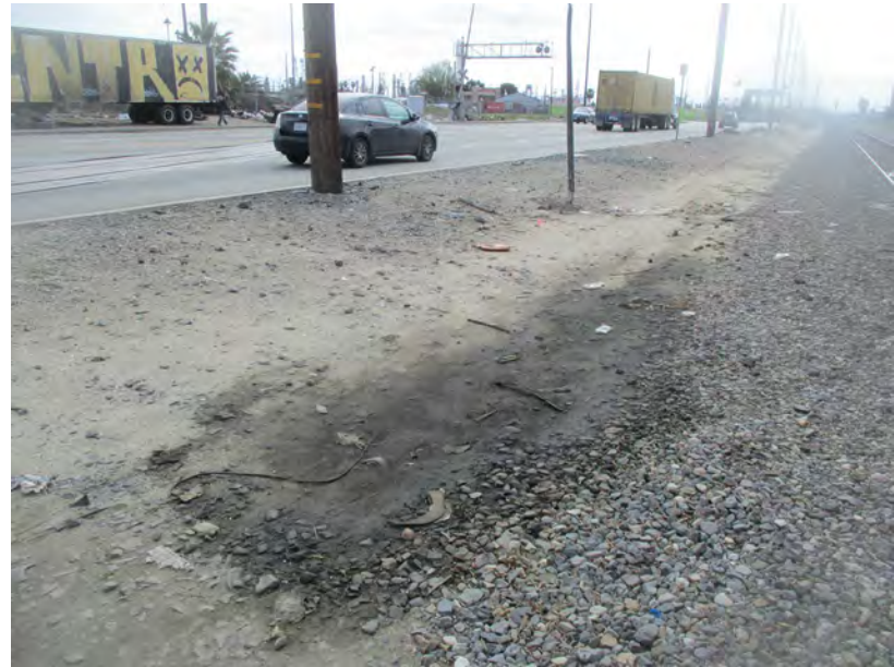
Oil stained area at north end of PHL railroad across from Valero Entrance.
