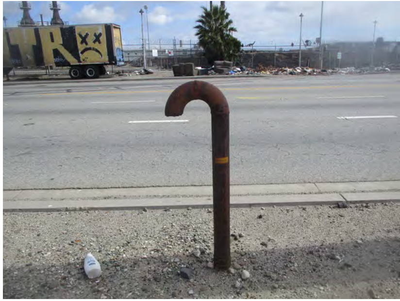
Pipeline vent pipe throughout PHL.
