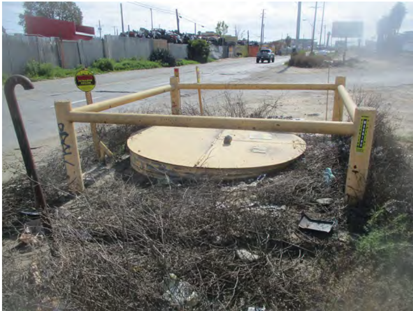
Pipeline vault at east side of PHL railroad.
