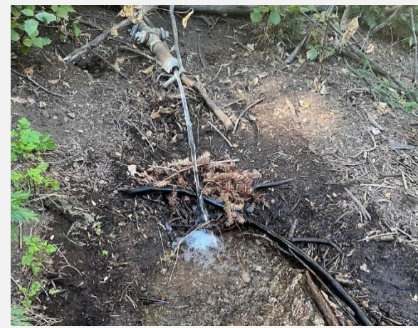
Photo 4. View of seep at top (southernmost end) of NWW-1. Photo facing southwest.
