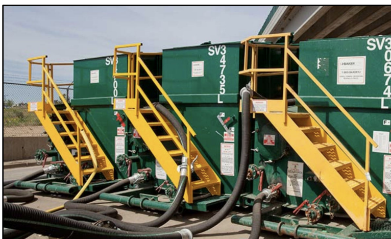
Figure 3. Example of Temporary Storage Tanks
