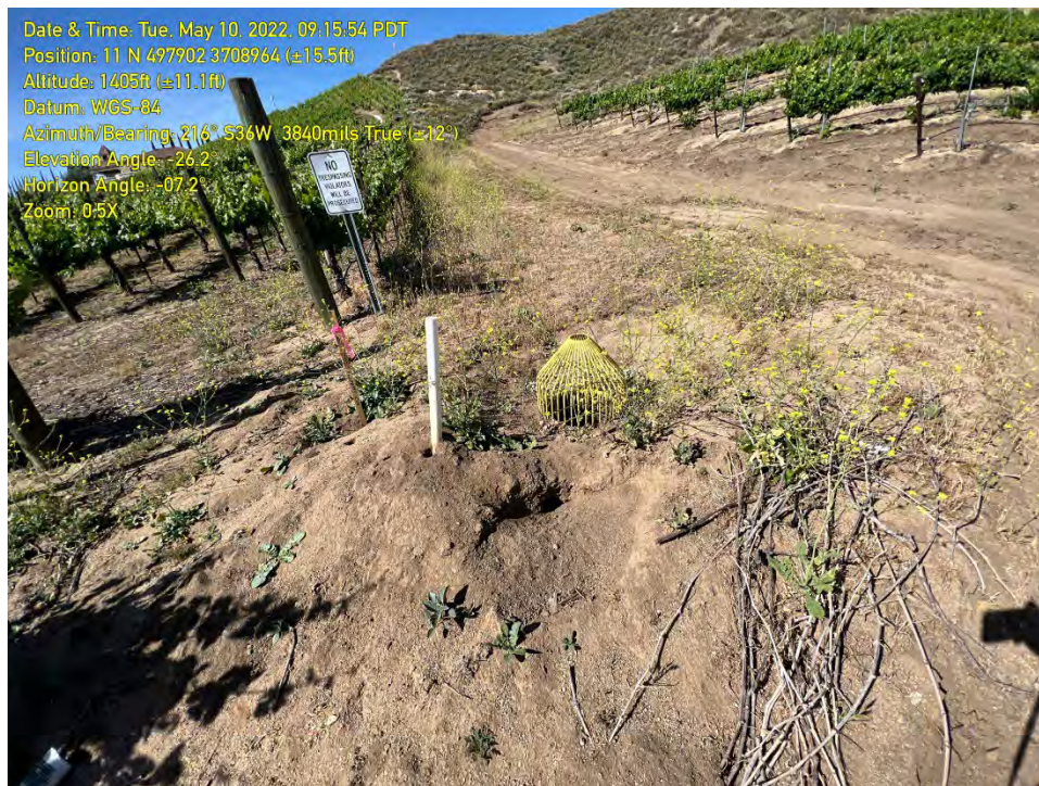
PHOTO 14: A drain in the central portion of the Site that conveyed stormflow underground via pipe to Feature A.
