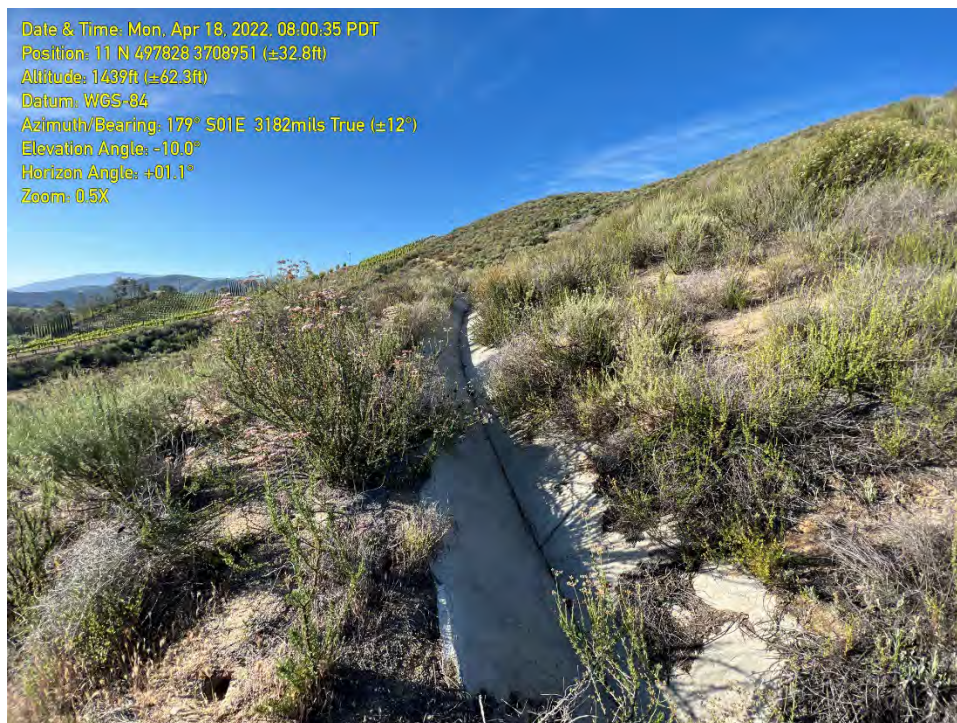
PHOTO 12: A portion of one of the brow ditches installed around 2007 to collect sheetflow to protect the vineyard and control erosion.
