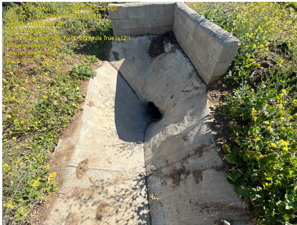
PHOTO 13: The culvert at the terminus of the existing brow ditch system where stormflow was conveyed underground via pipe to Feature A.
