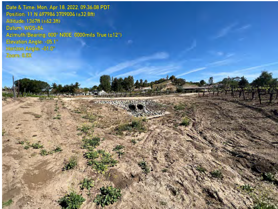
PHOTO 7: The downstream side of the dirt road depicting the concrete rip/rap and encased culverts.
