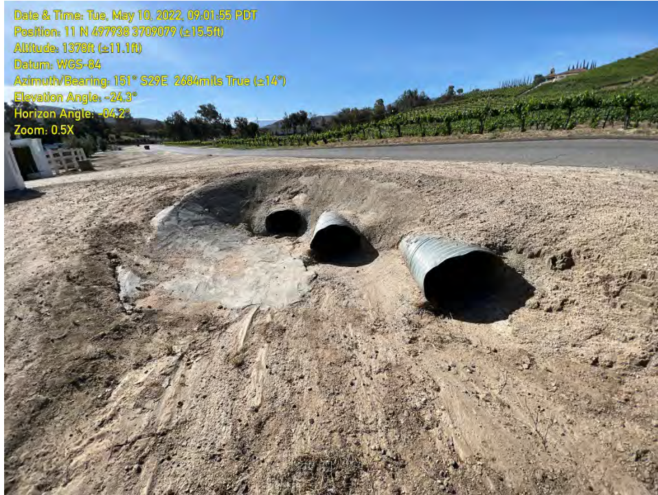
PHOTO 9: Three culverts north of Camino del Vino that convey Feature A storm flows onto the Property.
