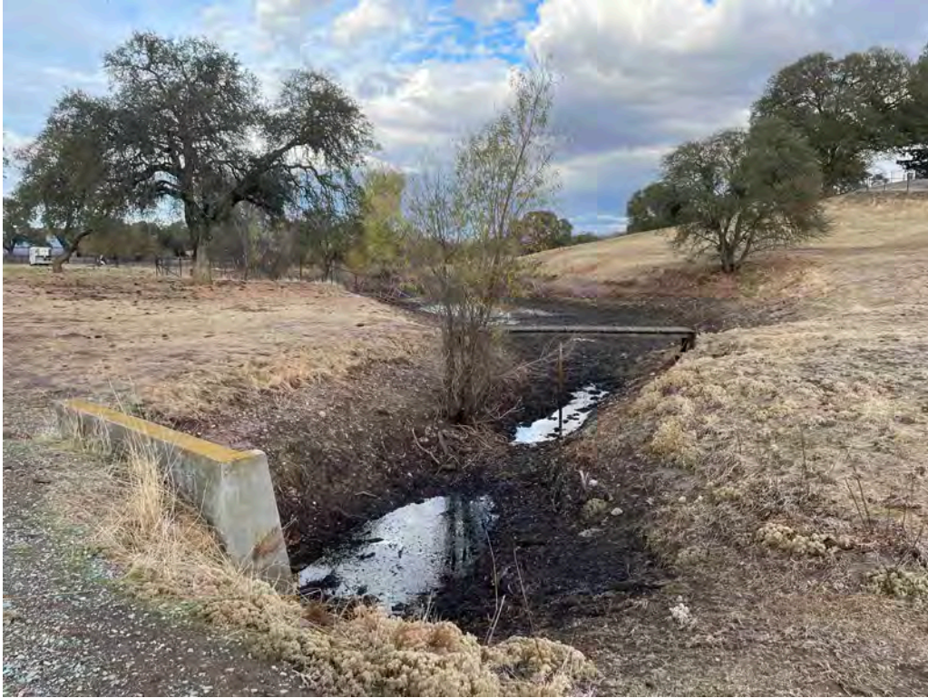
Stream crossing underneath the existing access road to the tower site. Water ponds in the area in center of photo. View looking east from access road.
