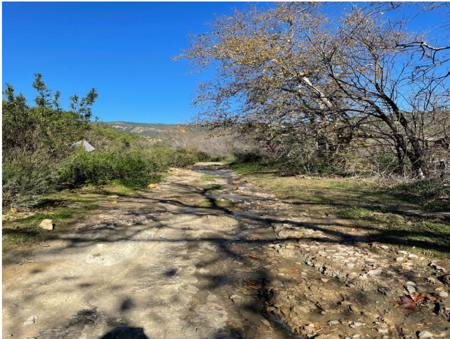
Access road past the vehicle bridge with erosion and water flowing down the roadway (January 9, 2026).
