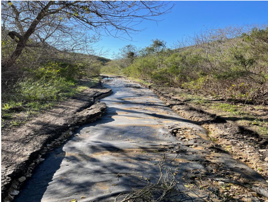
Eroded access road north of the second access gate (January 9, 2026).
