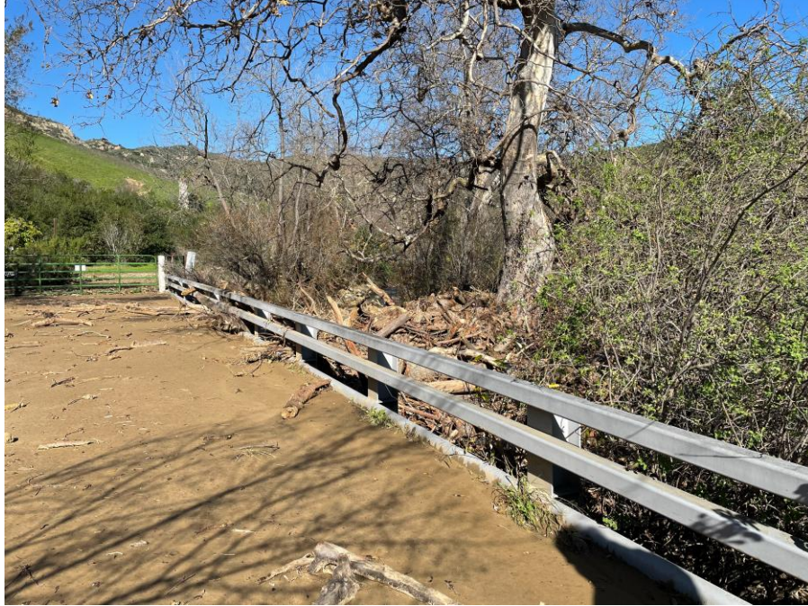
Vehicle bridge covered with silt, with debris lodged upstream and beneath the bridge (January 9, 2026).
