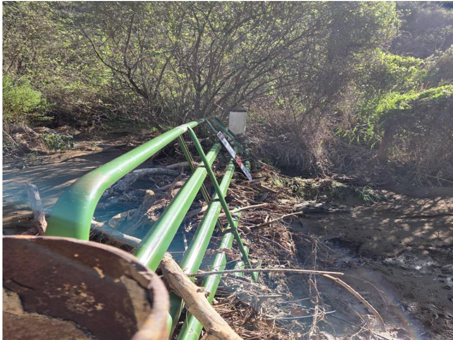
Second access gate with debris impact causing gate deformation (January 9, 2026).
