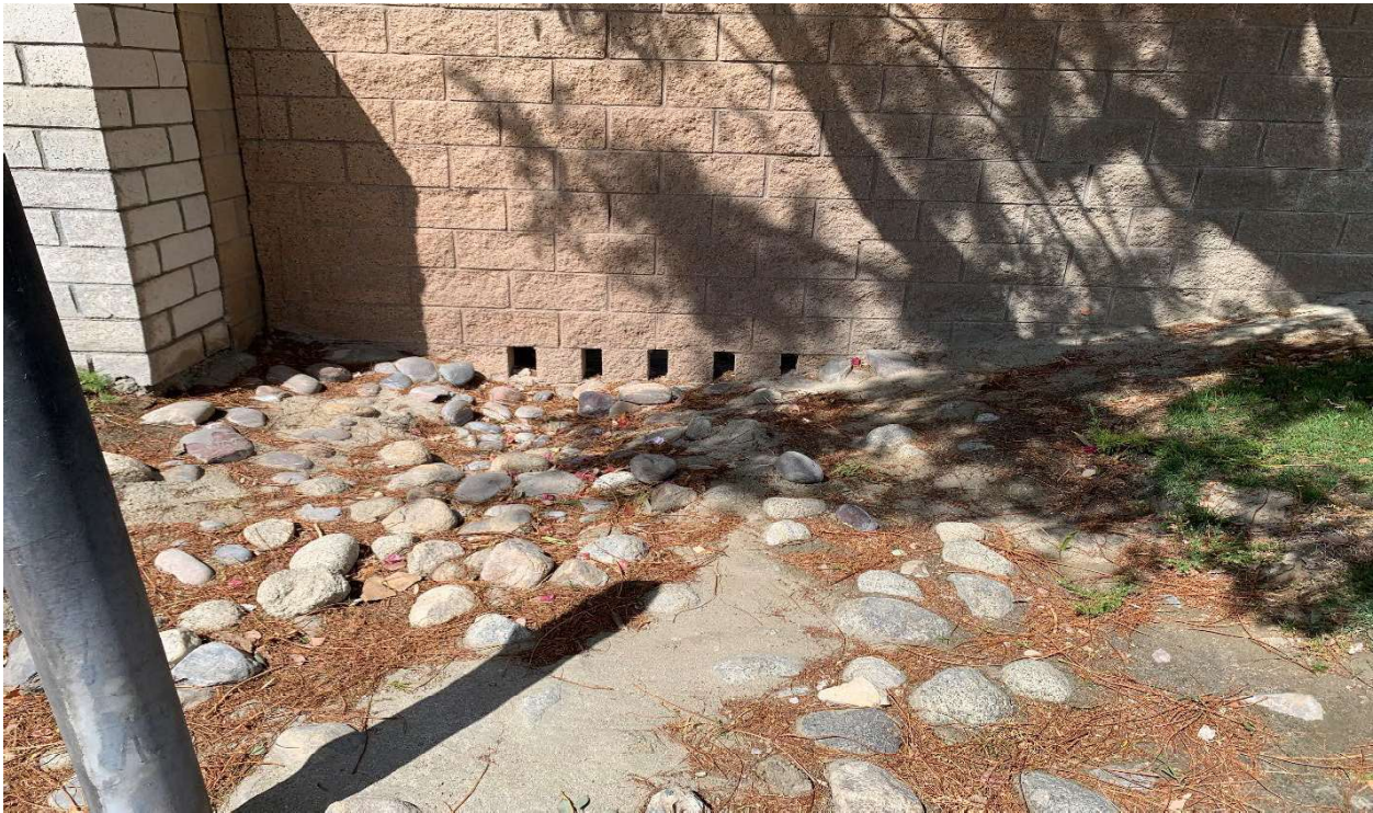
Photograph 9. View of ungrouted riprap on east side of brick wall with five gaps in the wall shown.
