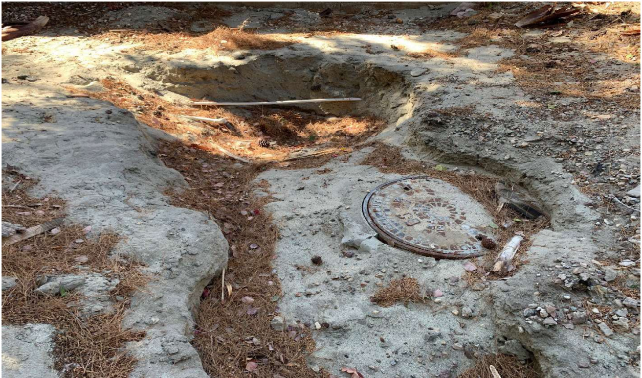
Photograph 5. Eroded area with man-hole and exposed PVC pipe at southwest corner of retention basin.
