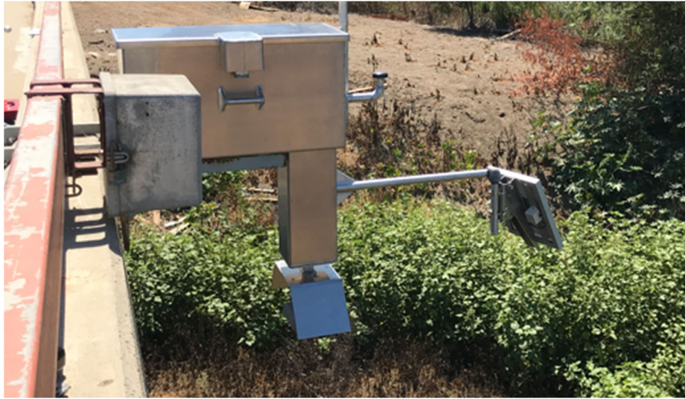
Photo from Ridgeview gaging location to show example of radar installation. The smaller box in front left is not part of the radar box.
