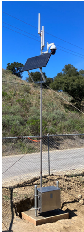
Photo from Arundell Camera location to show example of camera installation & concrete base.
