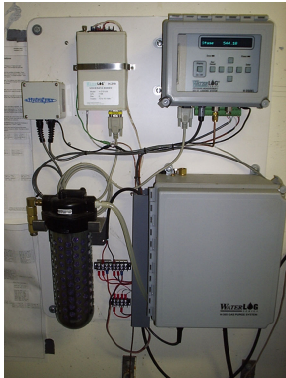
Photo showing current system at Lake Casitas which is inside the dam house mounted on the wall.
