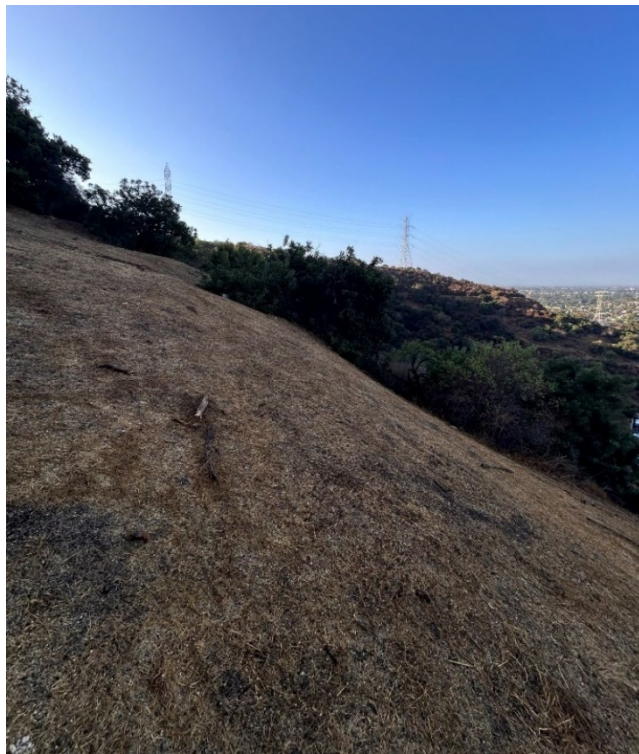
Photo 12: Open/disturbed area on northwest slope facing west.
