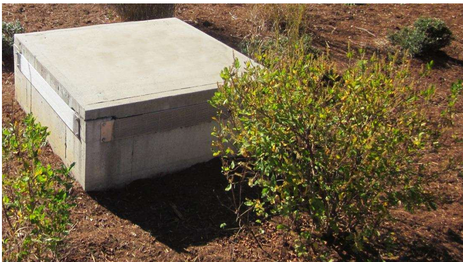
Figure 5. Outlet structure with a 5mm screen.
