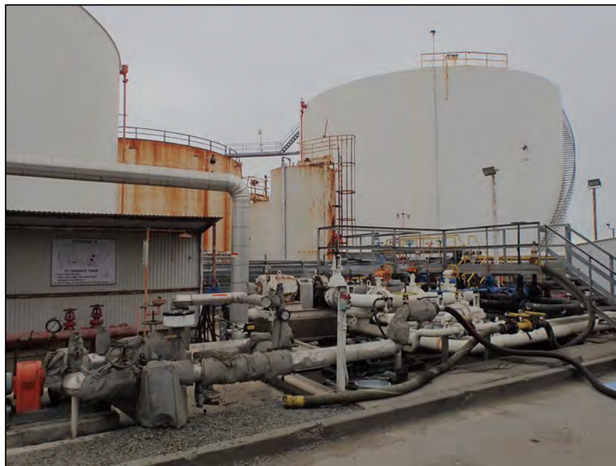
488 Wright Avenue. Tanks, piping, and fire suppression infrastructure, Representative view. View southeast. LSA photograph 9/26/24.
