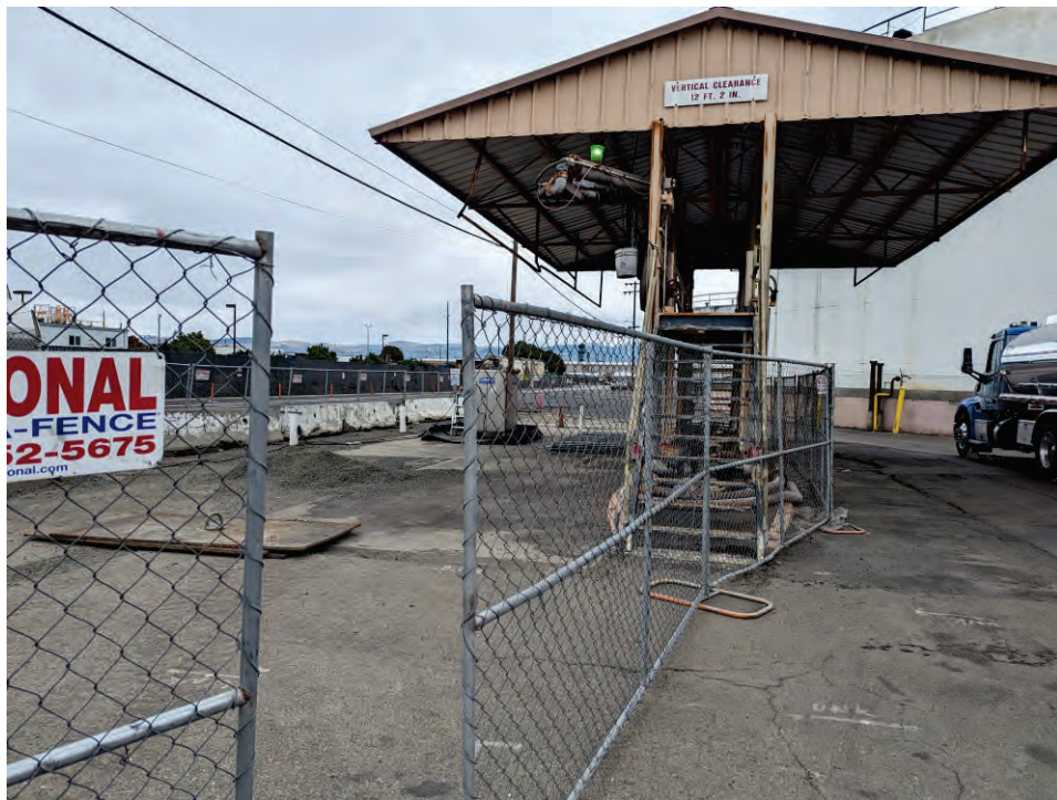
Existing Truck Rack
