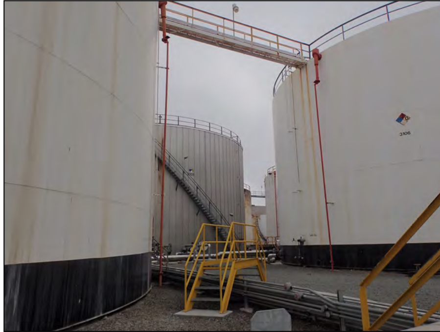
488 Wright Avenue. Tanks and piping infrastructure, Representative view. View southeast. LSA photograph 9/26/24.
