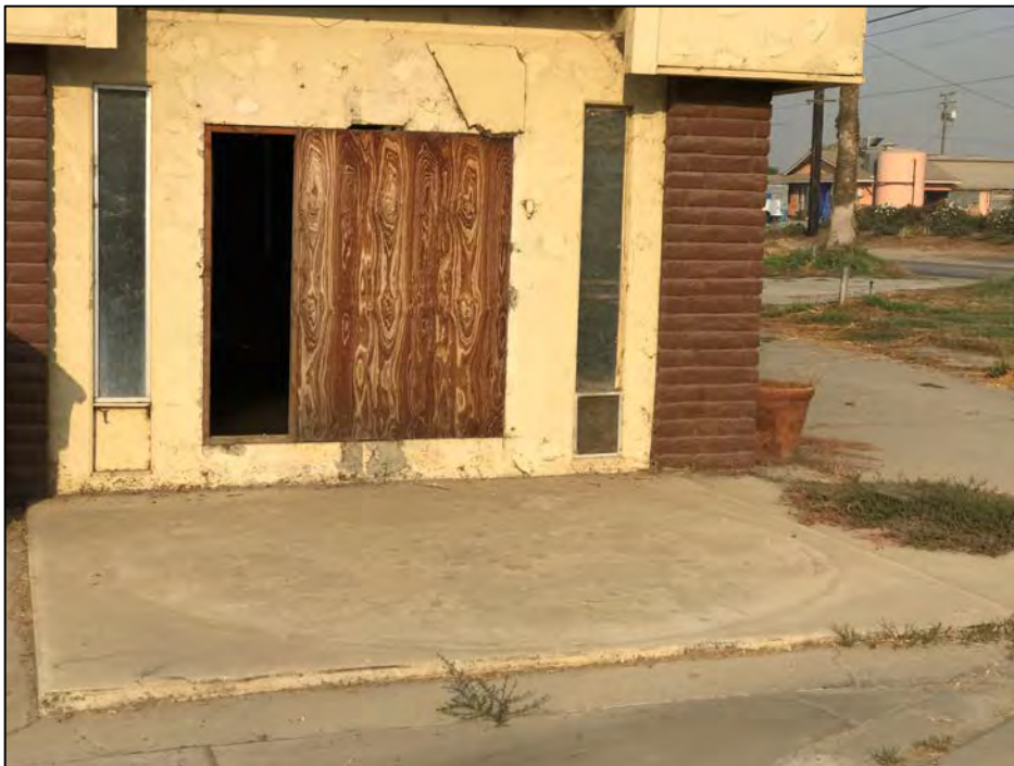
Close-up view of a boarded window and the narrow fixed pane windows. Source: VCS Environmental.
