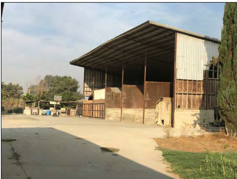
Close-up view of the ancillary pole structure. Source: VCS Environmental.
