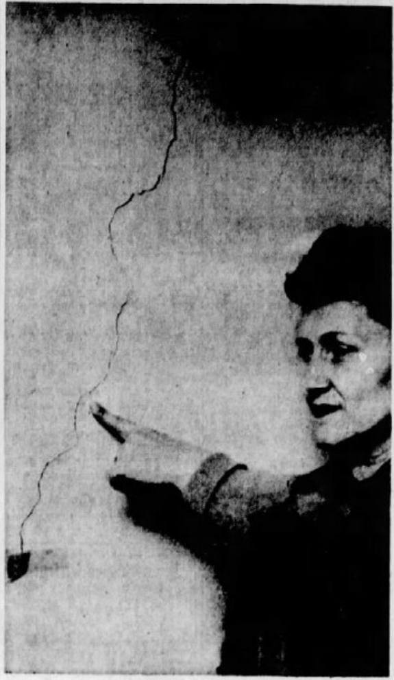
FIGURE 25 PHOTOGRAPH OF ONE OF THE CONCERNING CRACKS IN THE OLD COURTHOUSE AMIDST NEW COURTHOUSE EXCAVATION. ("INSPECTOR EYES COURTHOUSE CRACKS; WORKER MOVES," RECORD-SEARCHLIGHT , DECEMBER 9, 1954.)
