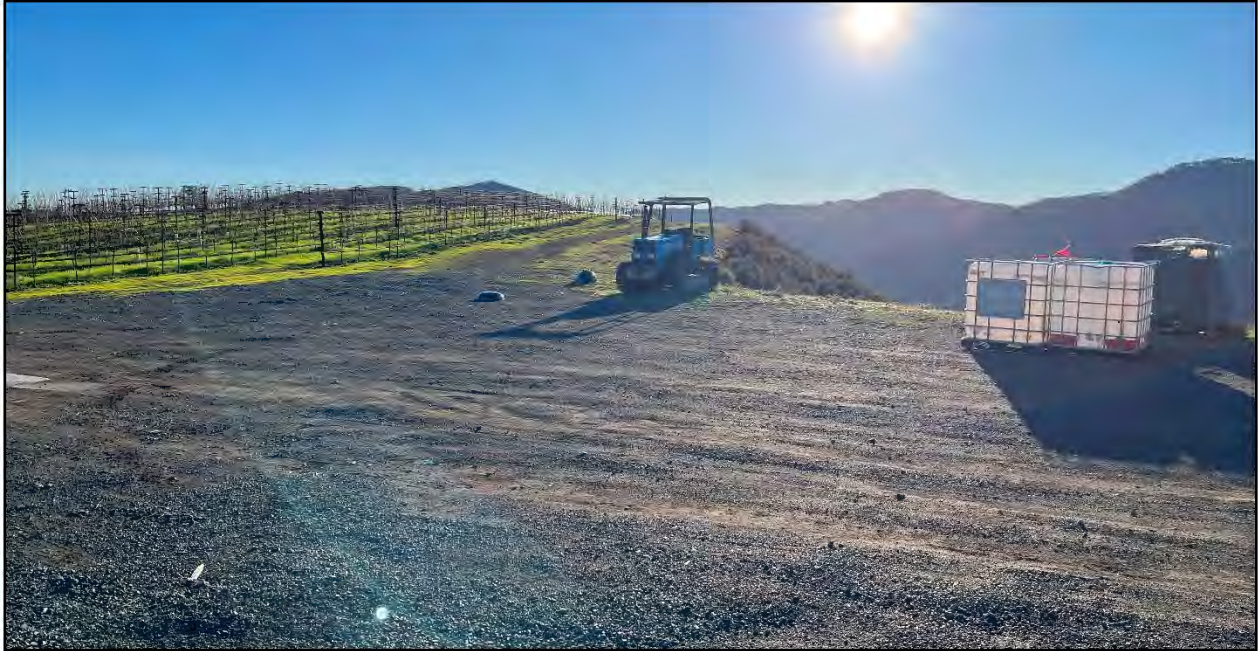
Paul's Well (PW) potential spoils area supporting developed areas with adjacent native trees (coast live oak); earthen spoils would be deposited and spread out with light to medium machinery
