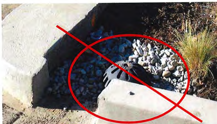
Figure 6: Incorrect Placement of an Overflow Inlet.
