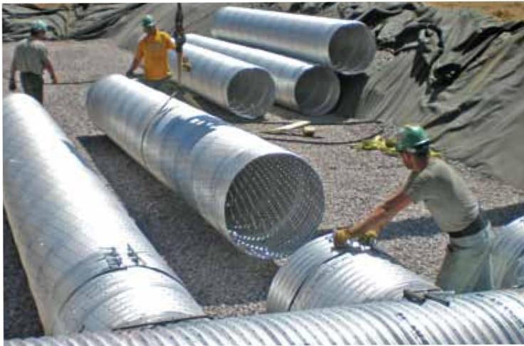
Perforated CMP infiltration system
