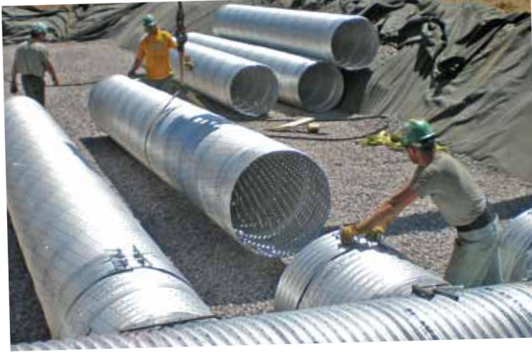
Perforated CMP infiltration system
