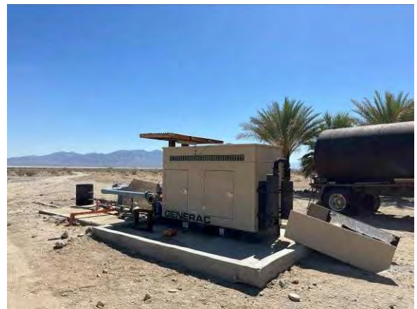
Photo #16 View of a generator with a diesel belly tank in the water pump area.
