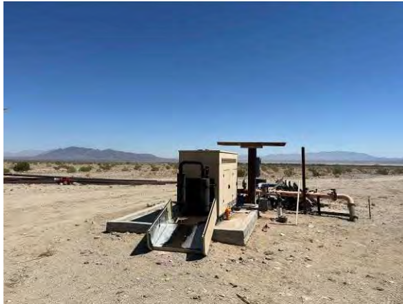
Photo #19 View of additional generator with diesel belly tank and water pump in the water pump area.
