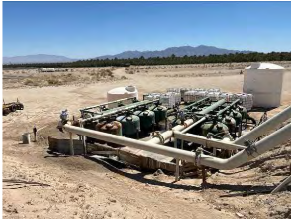
Photo #7 View of the water treatment system for the retention pond with ASTs containing water solvents.
