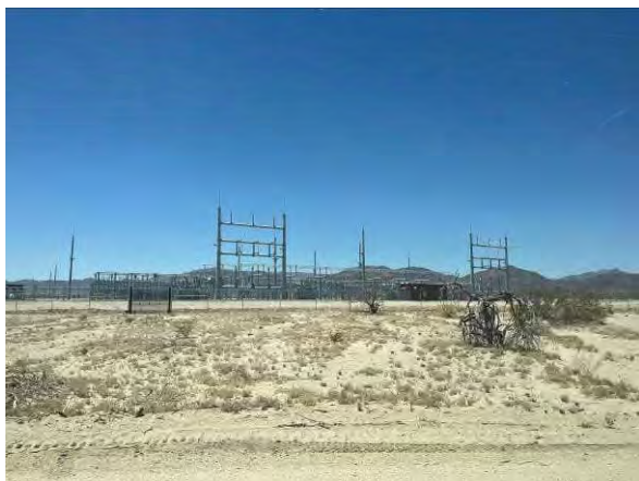
Photo #29 View of the adjoining substation that will connect the proposed gen-tie line.
