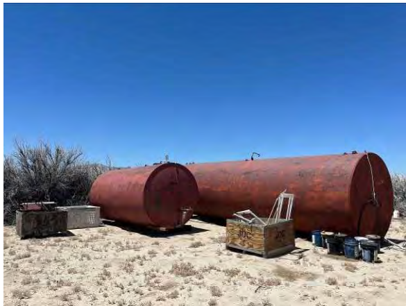
Photo #21 View of one 10,000-gallon diesel AST and one 20,000-gallon gasoline AST stored on dirt and equipment storage.
