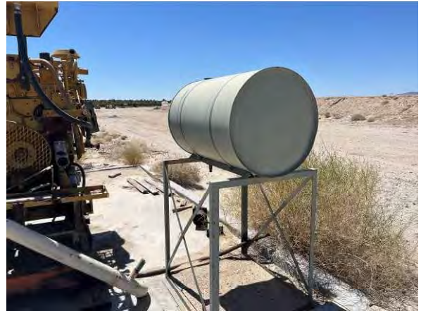
Photo #8 View of a 55-gallon AST of engine oil used for the retention pond water pumps.
