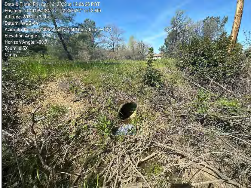
Photo 13. Showing the culvert that drains the larger wetland. Showing the culvert on the east side of Canby Road.
