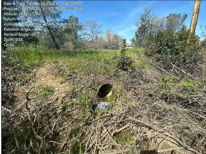
Photo 13. Showing the culvert that drains the larger wetland. Showing the culvert on the east side of Canby Road.
