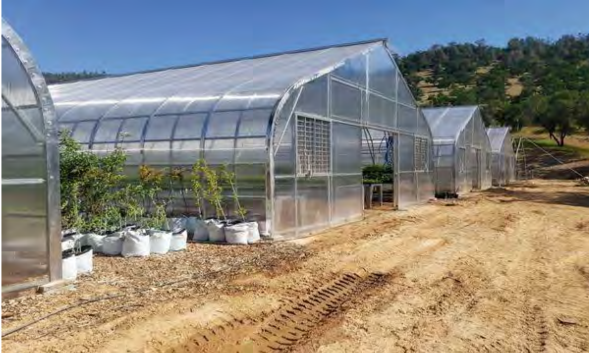
Photograph 13. Greenhouse area that once completed will have 18,000 square feet of greenhouse. Coordinates: 37.51449 °N, -120.01573 °W facing southwest. Photo taken by Mattole Whitaker on May 17, 2023.
