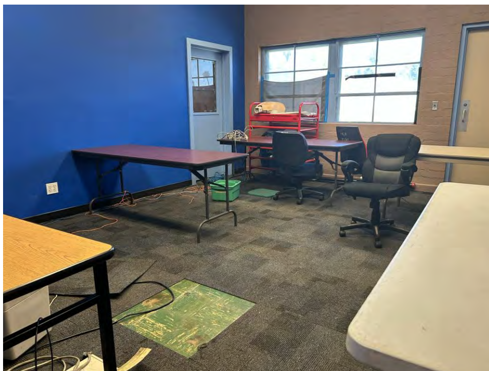
Figure 43. Interior of Mess Hall, view of old dining area. Asbestos tile visible under carpeted floor. View toward north.
