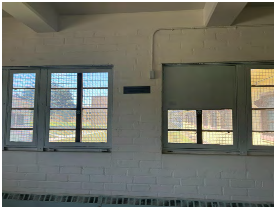
Photo 2. Detail of windows from the interior of dayroom. Windows have handles but have been bolted shut. View toward southwest.
