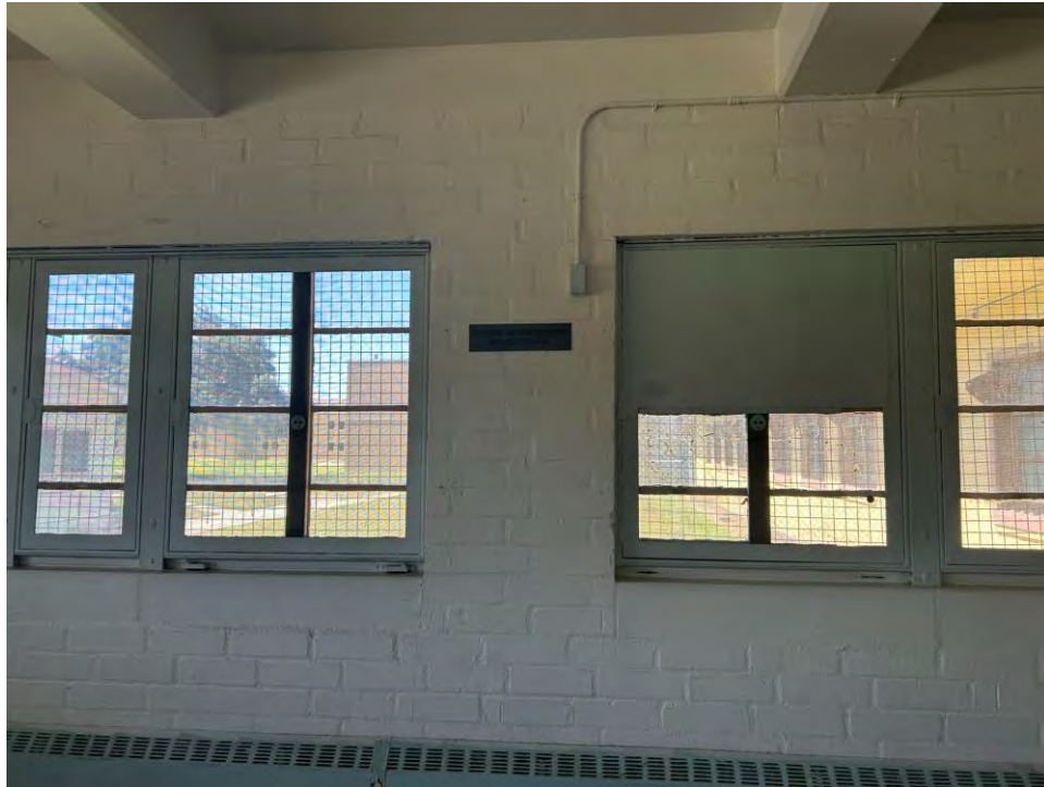
Figure 26. Detail of windows from the interior of dayroom. Windows have handles but have been bolted shut. View toward southwest.
