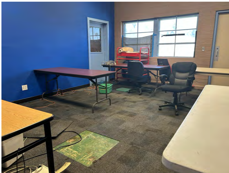
Photo 4. Interior of Mess Hall, view of old dining area. Asbestos tile visible under carpeted floor. View toward north.
