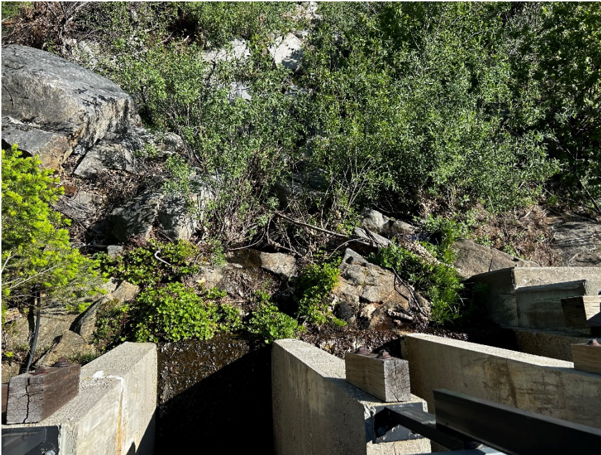
Photograph 1: View looking downslope flume abutment elevated above the area of the leak.
