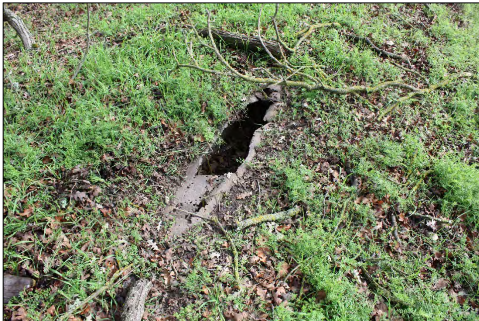
Photograph 3: Rusted through section of drainage pipe; facing east, February 8, 2024.
