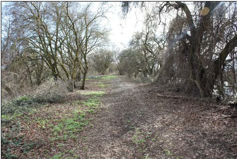
Photograph 11: North segment of Railroad Embankment, approximately 750 feet south of Twin Cities Road, showing uneven and irregular surface; facing south, February 8, 2024.
