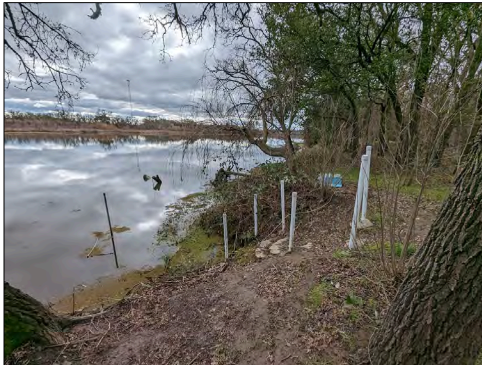
Photograph 17: Added informal dock and recreational features along the outer toe of the berm; facing southwest, February 8, 2024.
