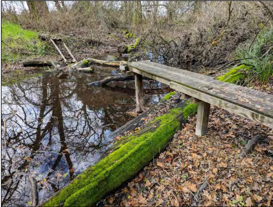
Photograph 4: A collapsed, modern footbridge previously spanned the slough near the west Property boundary; facing southwest, February 8, 2024.
