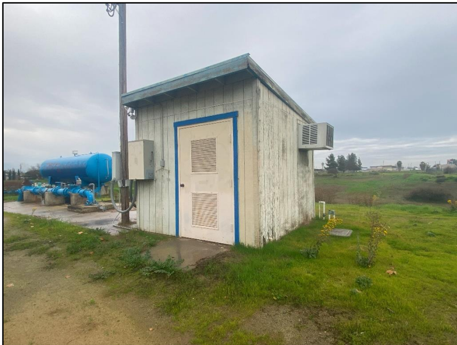
Figure 4-6 Well 11 and Tank, facing southeast.
