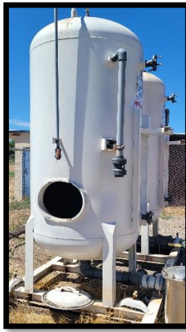
Photo 2: Looking Northwest at two tanks south of Well 02 near the eastern property line of Stanislaus Elementary School.
