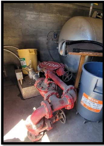
Photo 1: Looking West towards the existing SUSD-owned Well 02 near the eastern property line of Stanislaus Elementary School.
