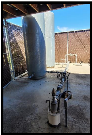
Photo 4: Looking Northeast towards Well 02 above ground appurtenances near the eastern property line of the School.
