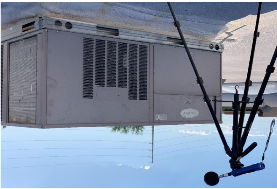
Figure 1: Commercial Air Conditioner - Carrier 50TFQ0006 - 5 Ton
