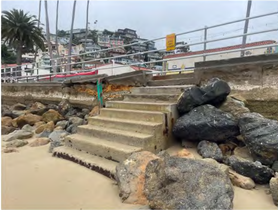
Photograph 4. Southernmost staircase showing signs of patchwork and previous repair efforts that were unsuccessful, view to southeast
