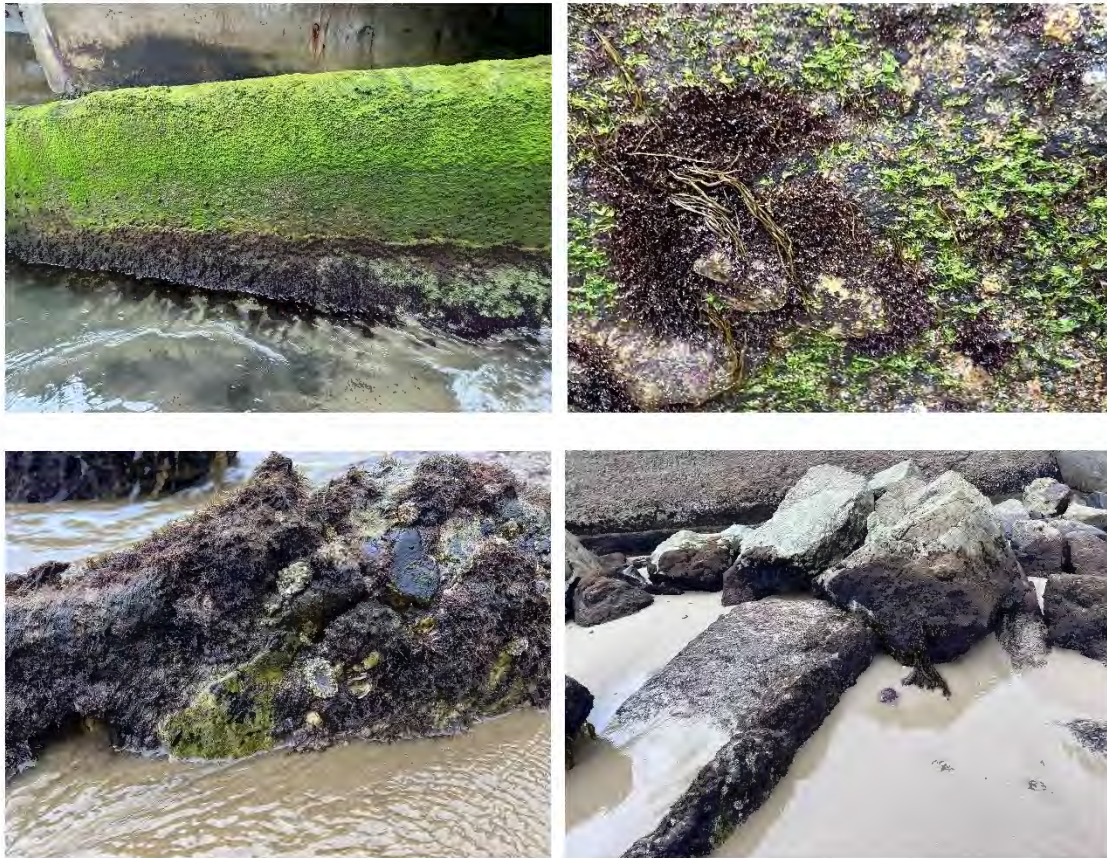
Figure 3. Photos showing examples of intertidal hard-substrate within the Project area. Bottom right photo shows debris from failed groin wall.
